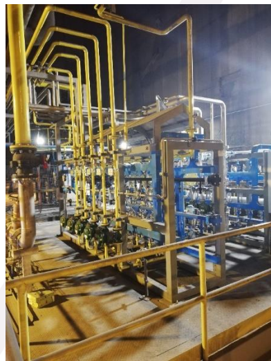
Fig 5 MORE Full control Valve Trains (Celsa Group)
