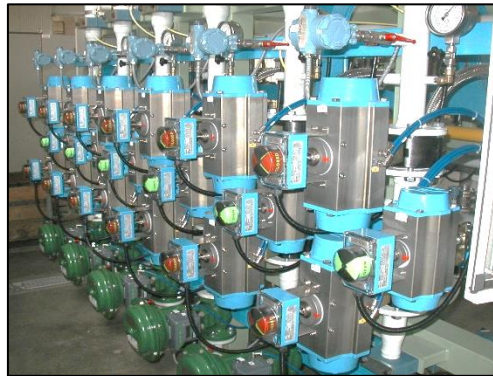
Fig 7 COG regulating valve train, Baosteel Shanghai No. 5 Steel Co. Ltd. (Baoshan, Shanghai, China)
