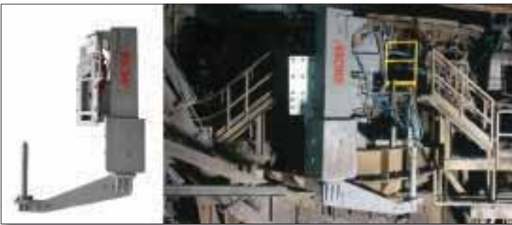
Fig 13 STROP in operation on an EAF in Mexico
